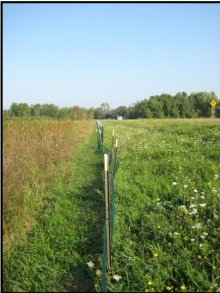
Images of installation of the SLRREF – supported wildlife fence project at Upper & Lower Lakes State Wildlife Management Area.
